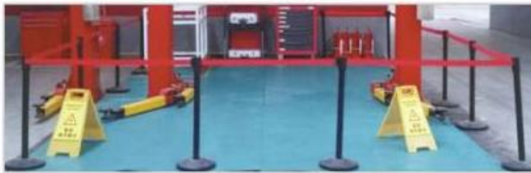
Fig 7-3 Safety isolation area
