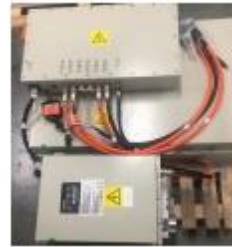
Fig 7-2 Orange high-voltage connection line
